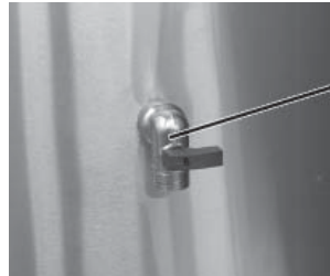
Control valve of steam generator
