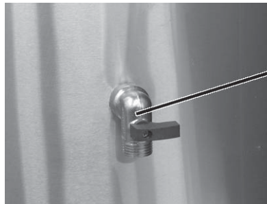
1. Control valve of steam jacket
